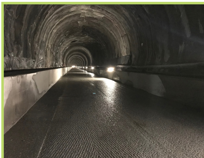
StreamLED Power - Osvetlenie tunela
